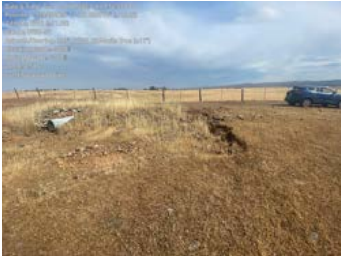
TH002737.JPG 13: overflow around pipe
