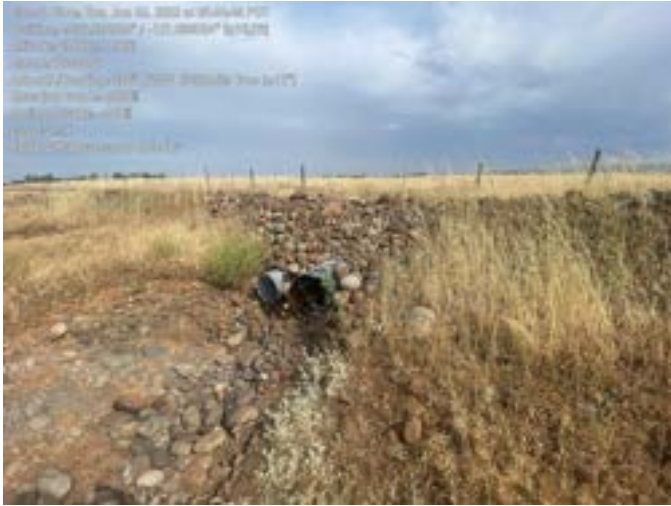
TH002731.JPG 7: ROAD 4 ft above scour hole inv
