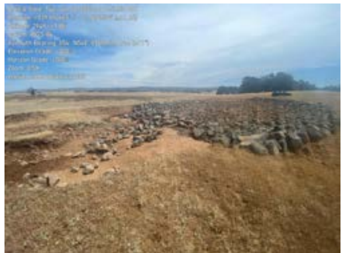
TH002838.JPG 114: erosion control spillway fail
