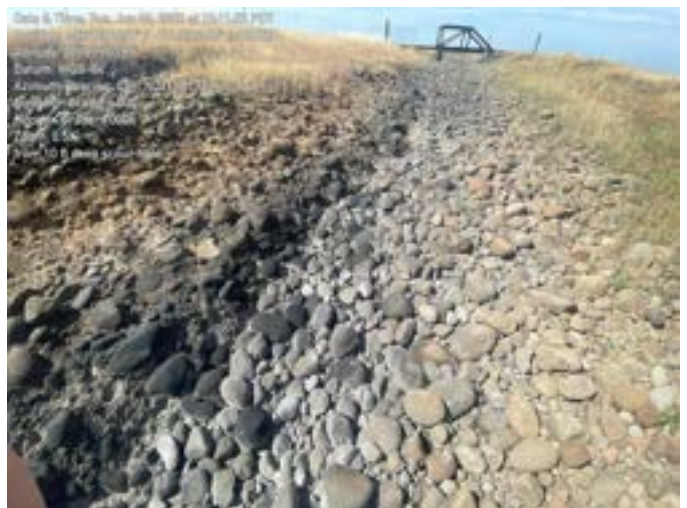
TH002760.JPG 36: from 10 ft deep scour hole
