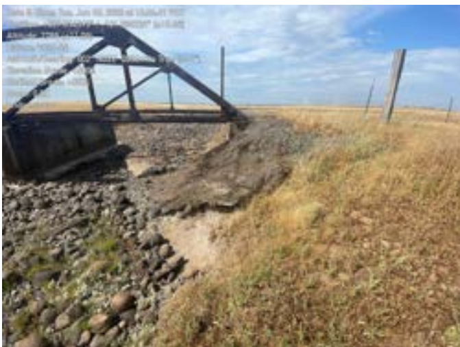
TH002753.JPG 29: bridge scour
