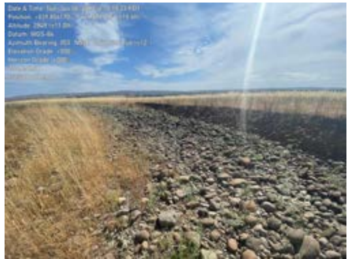
TH002774.JPG 50: erosion at bend
