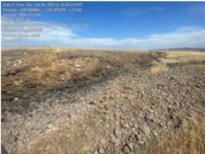
TH002793.JPG 69: scour 12 ft deep from bank
