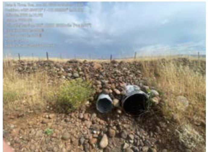
TH002730.JPG 6: ROAD 4 ft above scour hole inv
