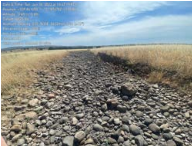
TH002811.JPG 87: bank erosion channel 20 wide
